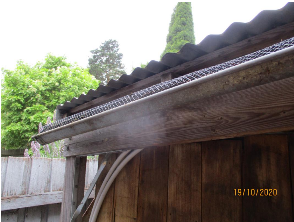
4. Properly support roof gutter of detached carport.
