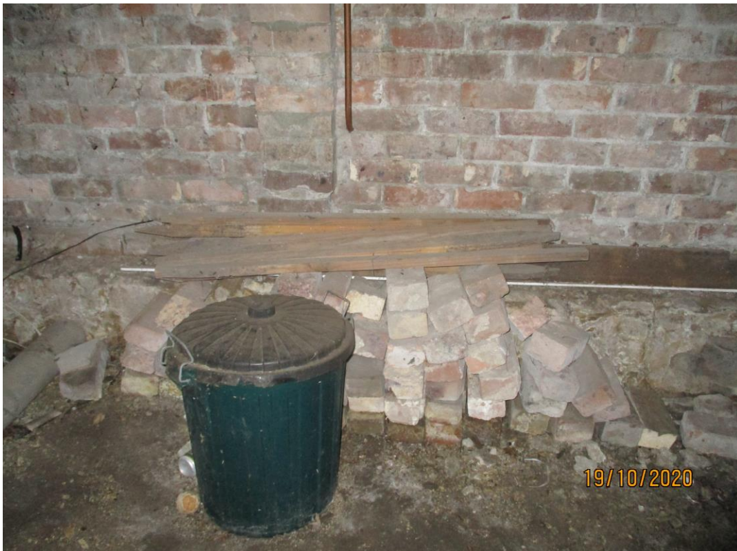
8. Significant amount of debris in the subfloor which will need to be removed
