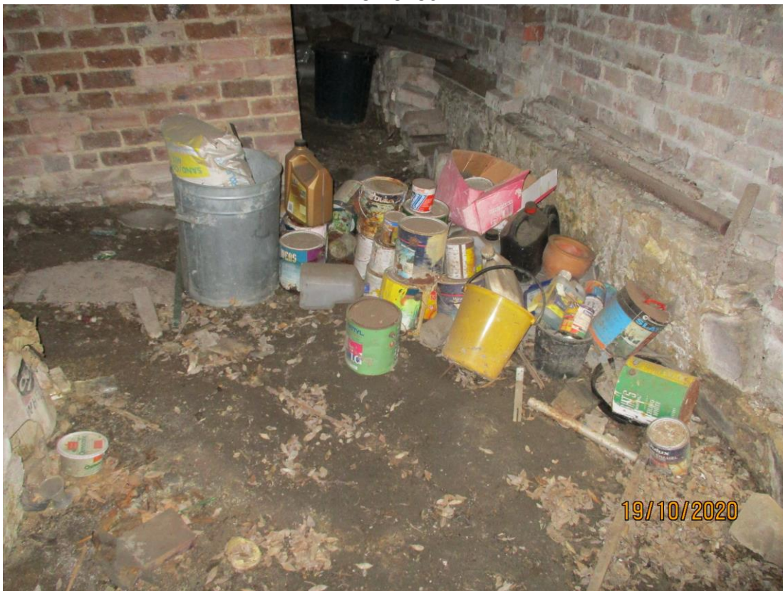
6. Significant amount of debris in the subfloor which will need to be removed
