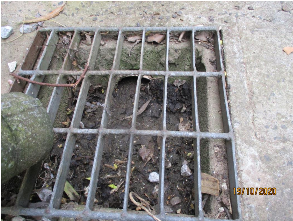
3. Clean out the stormwater pit and ensure that the stormwater is freely draining
