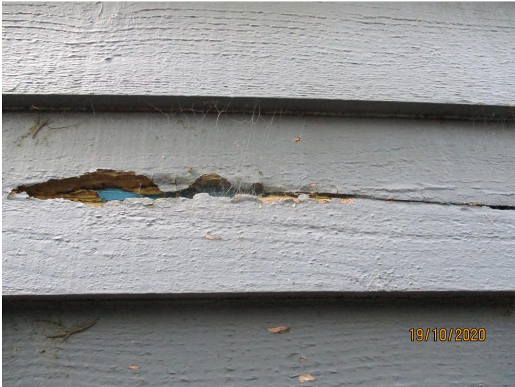
11. Some of the weatherboards have fungal decay which may allow the entry of moisture into the building
