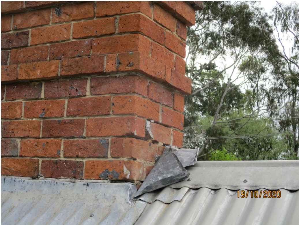
1. Repair the flashings to ensure that the chimney is weather-proof
