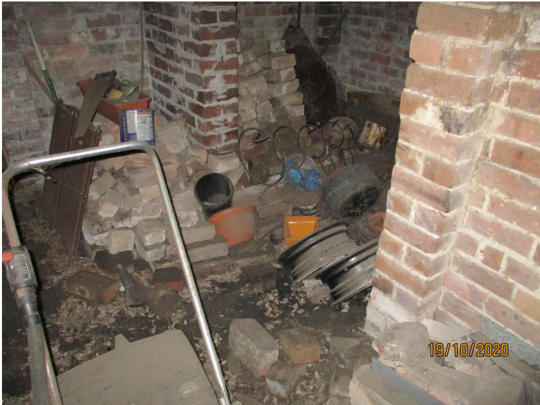
5. Significant amount of debris in the subfloor which will need to be removed
