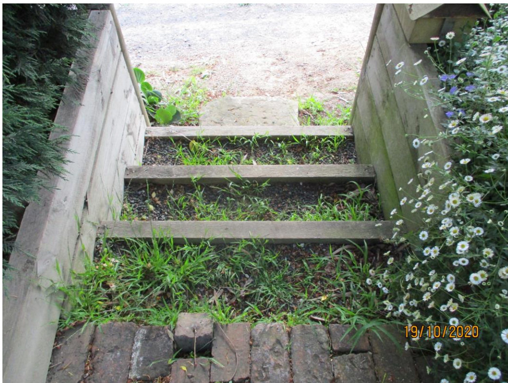
12. The front entry steps from the street footpath should be reformed for safe access in compliance with the Building Code.
